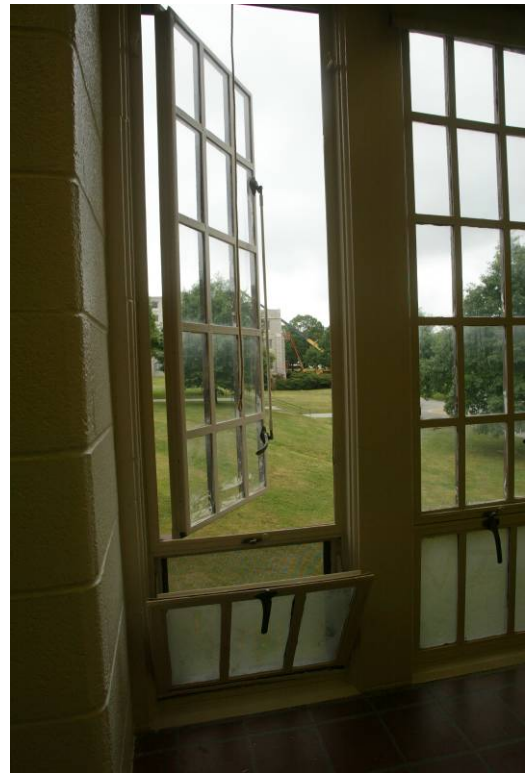
Figure 12. To Escape, They Had to Climb Over the Low Window
